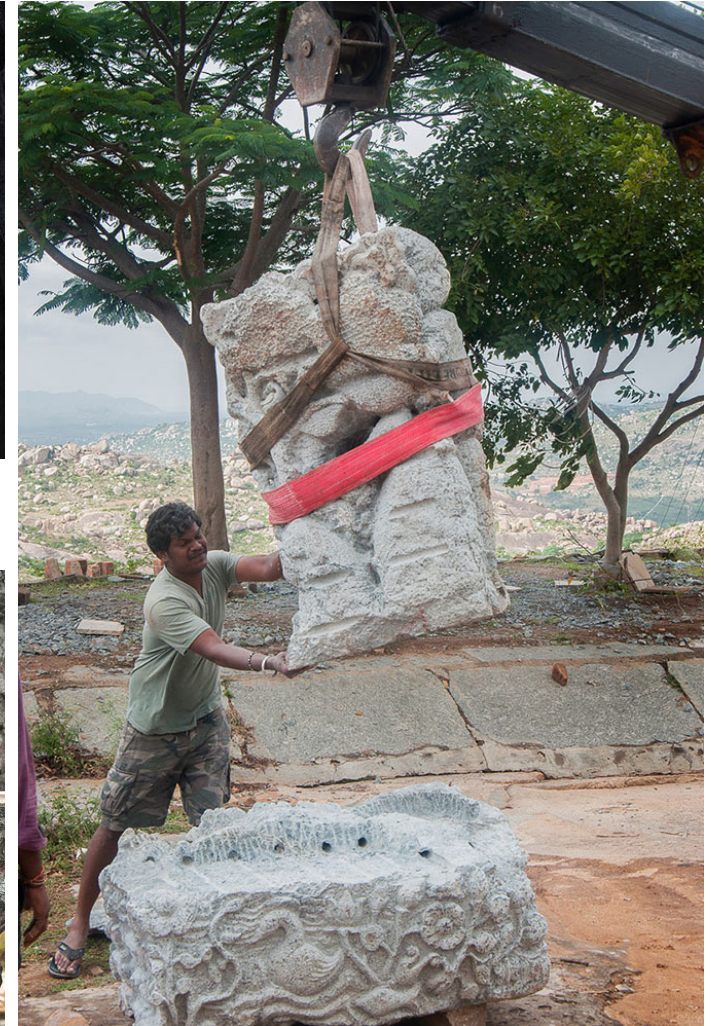
The process of installation of the sculpture is made with the help of crane.
