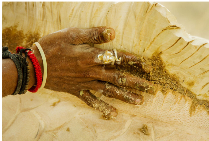
This mixer of wooden powder and adhesive agent are applied on the joints and cracks.
