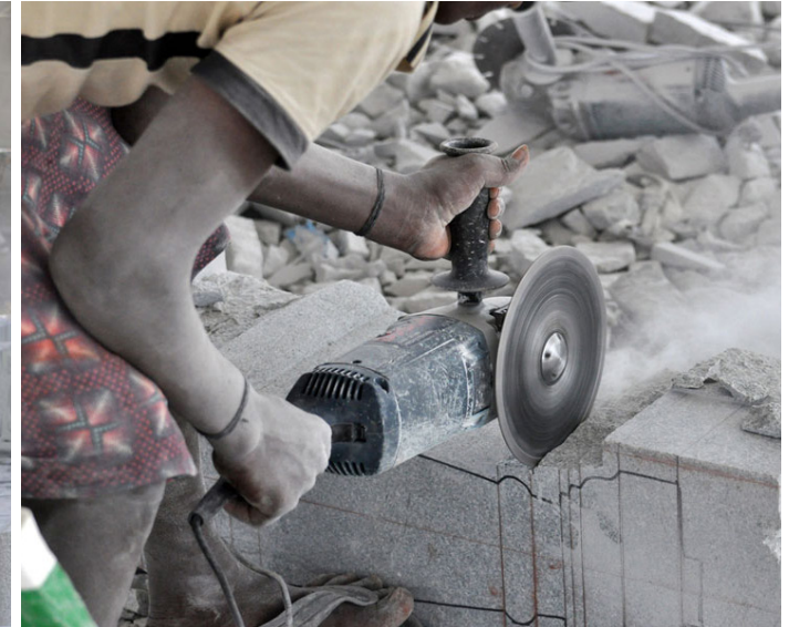
The master craftsmen divide the work of sculpting into the three parts depending on the shape and size of the structure to be made.
