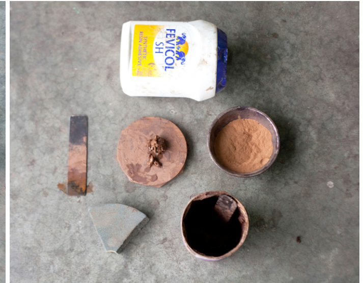
After rubbing the surface with stone, Fevicol, and saw dust is mixed together to make putty. This putty is applied using the metal strip.
