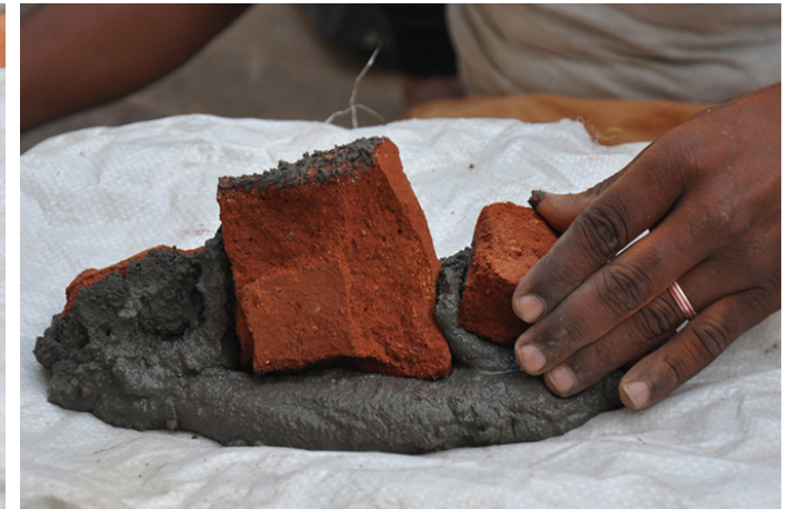
Few bricks are placed on the thick layer of cement according to the sculpture.
