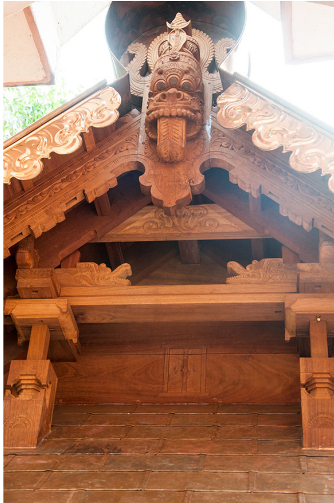
The detailed wooden vyali on the top of the roof is made and installed.
