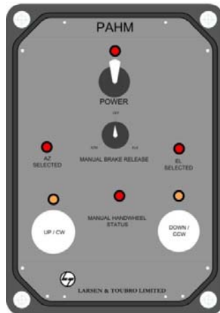
Control Panel and old PAHM module
