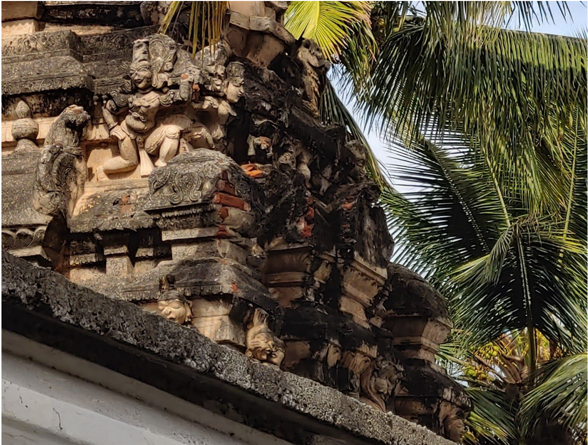
Figure 19. Small size bricks are visible in the cracks in vimana.
