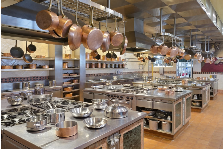
Figure 1: A typical commercial kitchen
