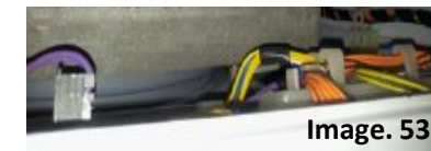
Connections for control panel
