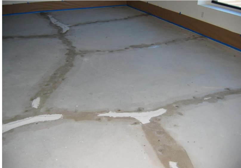
Fig.16 Damage to traditional cement flooring http://www.madstonefloors.com/wp-content/uploads/2011/02/IMG_4454.jpg seen as in 12/11/2014
