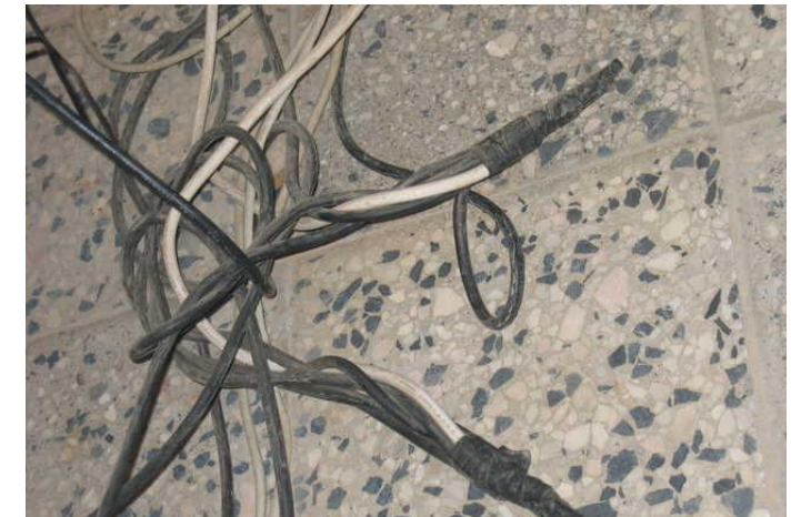
Fig.25 (c) computer wiring http://alexlittle.net/blog/images/2008/12/img_3119.jpg as seen on 11/10/2014
