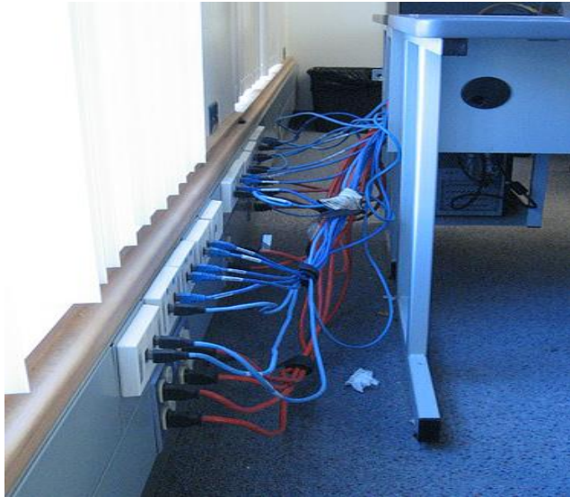
Fig 25 (a) Communication cables https://c1.staticflickr.com/1/42/102017268_756ae32e41.jpg as seen on 10/11/2014
