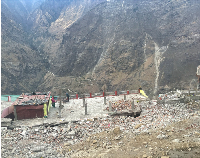
Fig 2.6 Issac, R. People set up a temporary structure in the debris of a demolished house. Joshimath. 2023.
