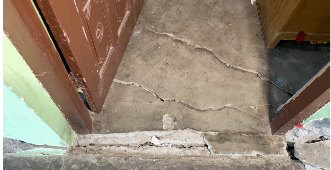
Fig 2.9 Issac, R., The cracked plinth of house marked for demolition. Joshimath. 2023.
