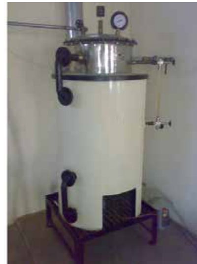
Fig6. Fire wood steam boiler
