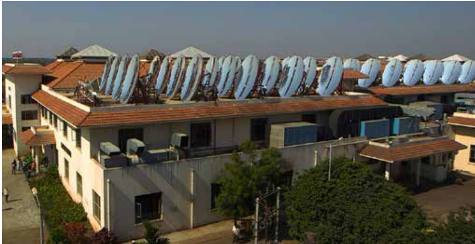
Fig20. Solar receivers at Shirdi, Maharashtra
