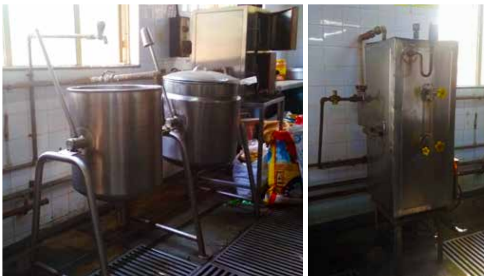
Fig22. Cooking vessel and steam boiler at hostel-6, IITB
