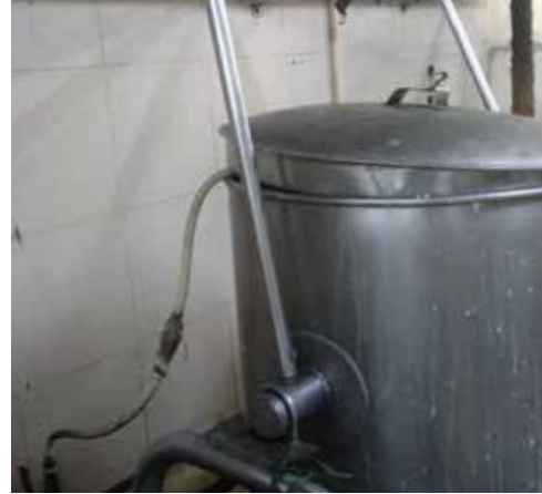
Fig25. Water inlet to vessel
