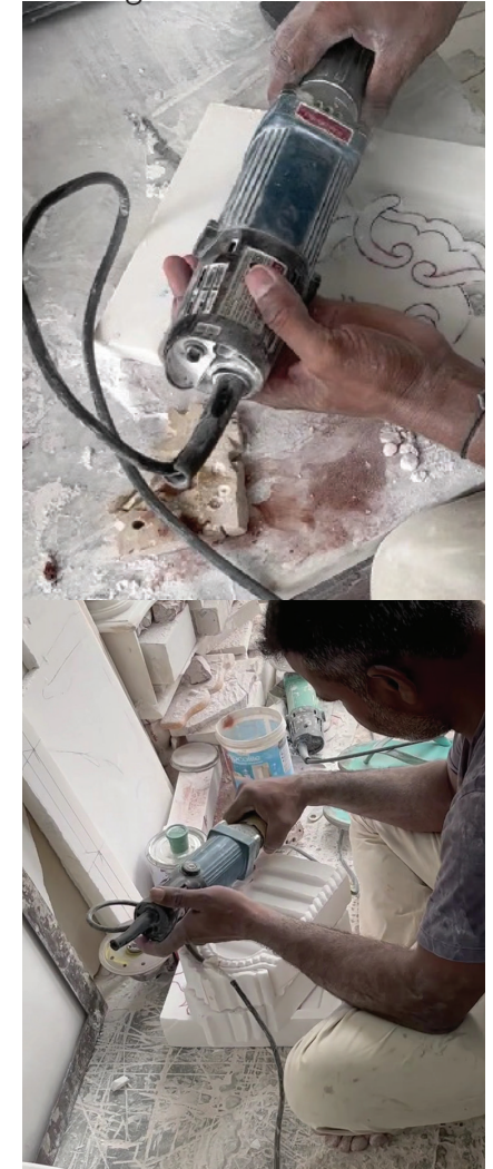
Fig 9.1.3: Dust Clearing Provision
