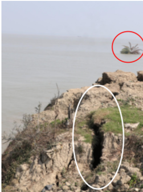
The crack demarcates the part of shoreline that will soon wash away. At a distance, a datepalm tree is seen which was previously above sea level
