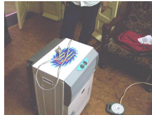
Wire is left open
