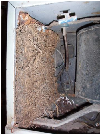
Side and rear panels covered with dry grass
