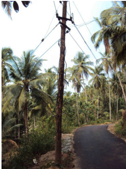
Figure 3-31. Electric lines in narrow road [32]
