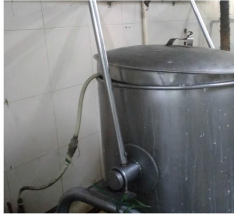
Water inlet to vessel
