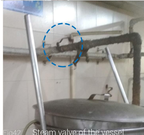
Fig42. Steam valve of the vessel.
