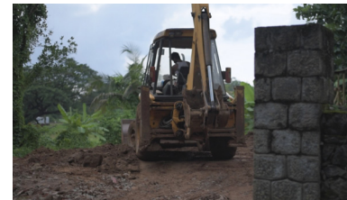
Old buildings and paddy farms are razed down to make space for new apartment buildings.
