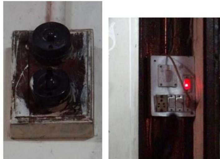
Details of old switches
