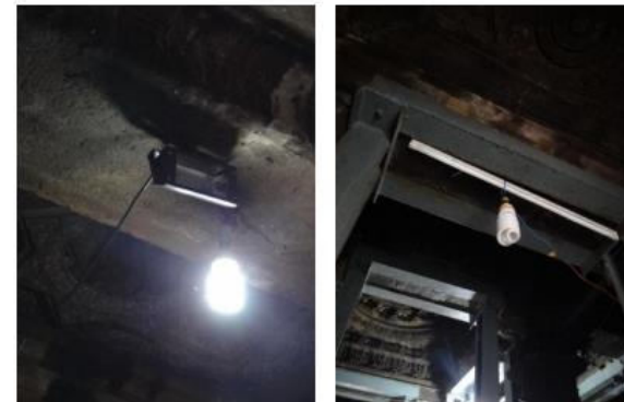
CFL bulbs hung on the porch and from the iron beam reinforcements
