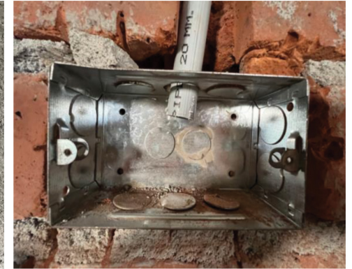
It needs to cut the wall according to the wiring path to install fitting and then it will be covered using concrete.
