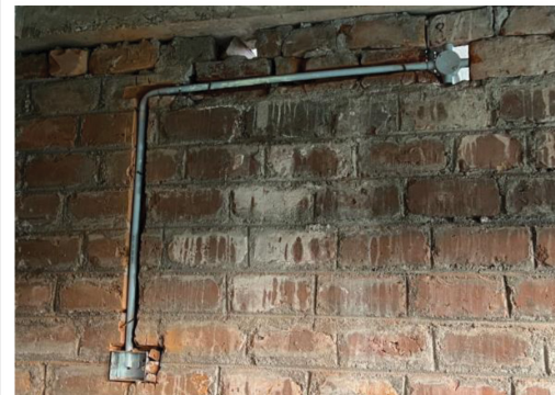
Concealed wiring and joints.
