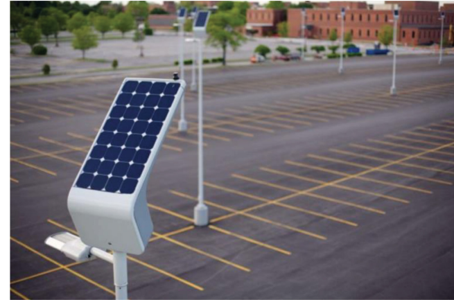
Image 30 – parking lot lights
