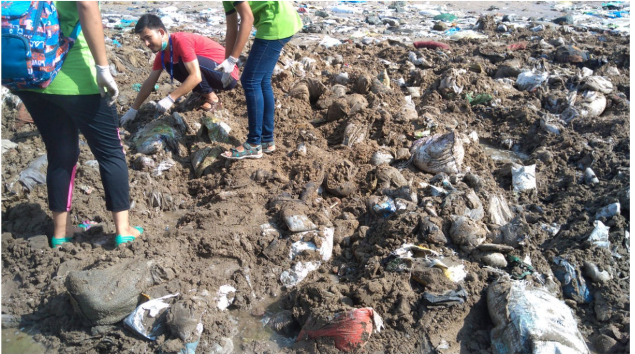
Image 35: Volunteers need to walk over the dug-outs and manually pull out the heavy sand bags
