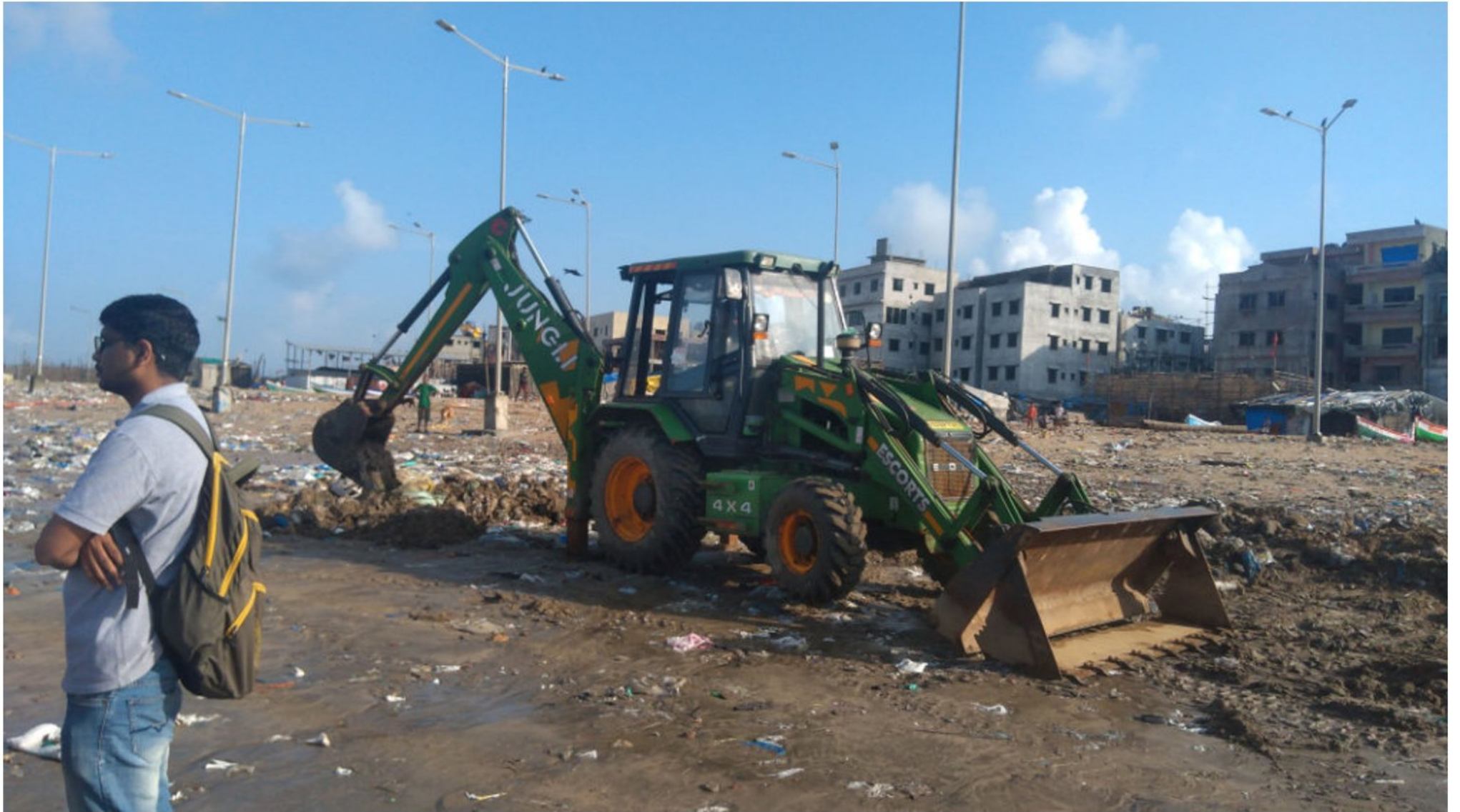
Image 34: Verova beach is provided with diggers and earth movers to take out plastic bags from underground
