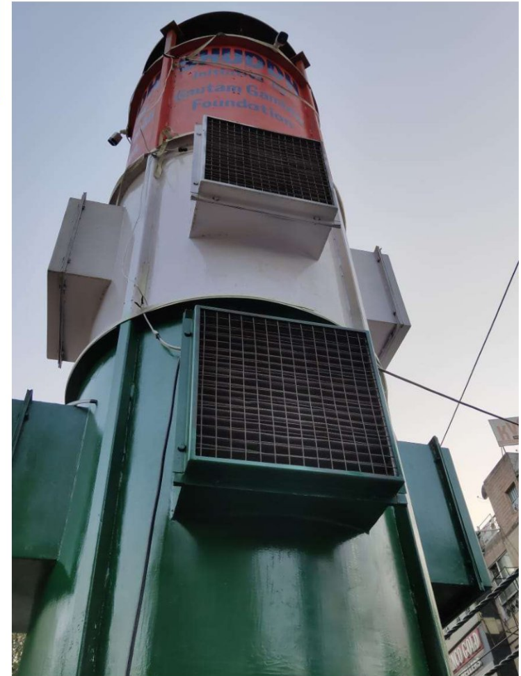
Smog tower installed in Lajpat nagar.
