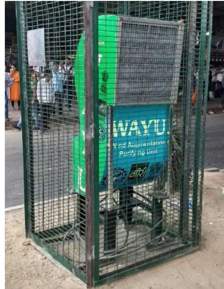
WAYU air purifier installed with a fence to protect it form public tempering.
