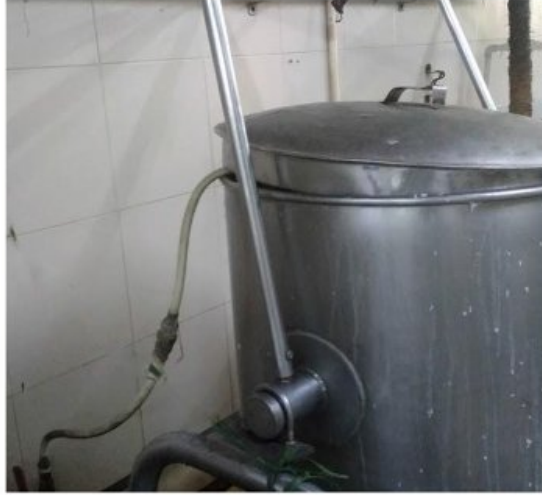
Water inlet to vessel
