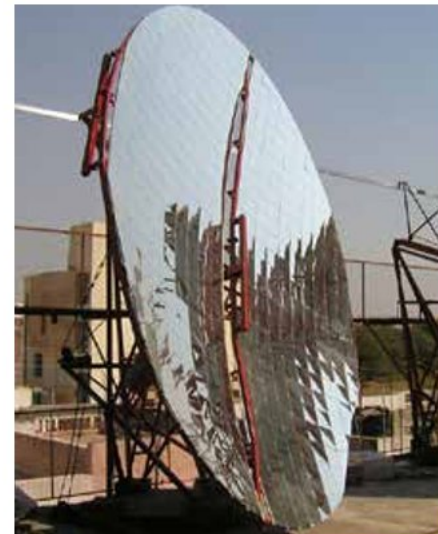
Fig7. Solar steam boiler
