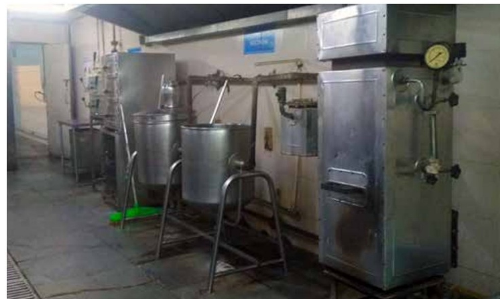
Fig23. Steam boiler and cooking vessel at hostel-12, IITB
