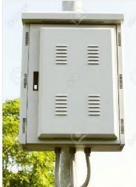
HRCA Outdoor Electric Panel Box. (Image source)
