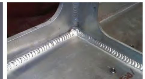
Weld Seam. (Image source)
