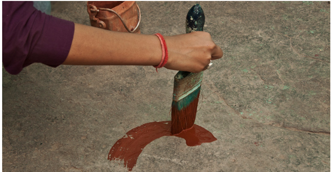
Geru (red clay solution) is applied on the floor as a base for the painting.
