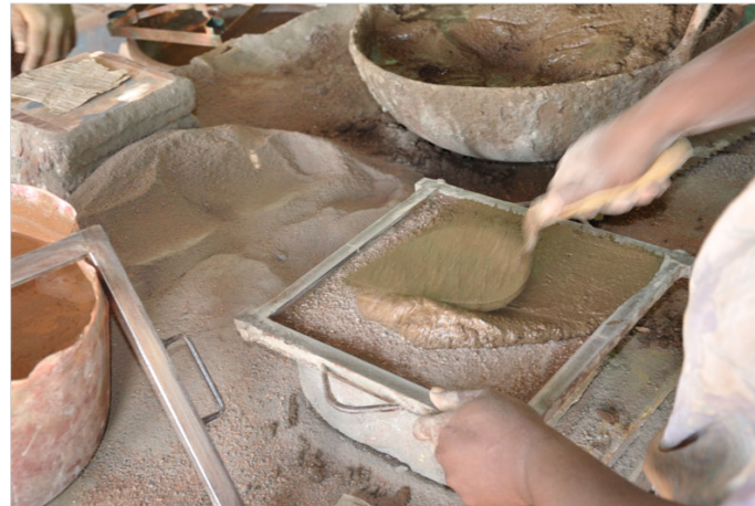
After a little drying mortar put and equally spread with the help of spade.
