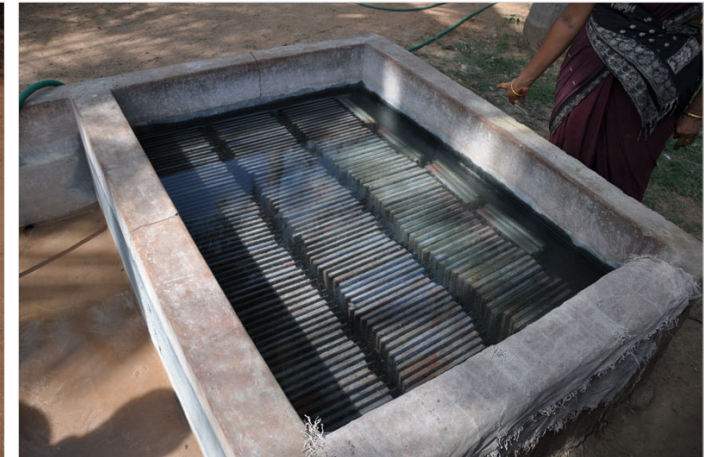
Once dried all the tiles are dipped in water tank to soak water (curing) and avoid breakage.
