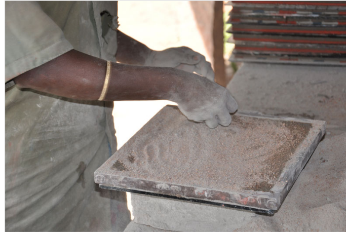
Dry cement and sand is added to fill the gaps and then leveled.
