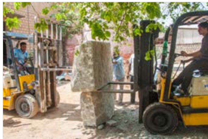
Later the stones are placed one on the other vertically with the help of forklift trucks.
