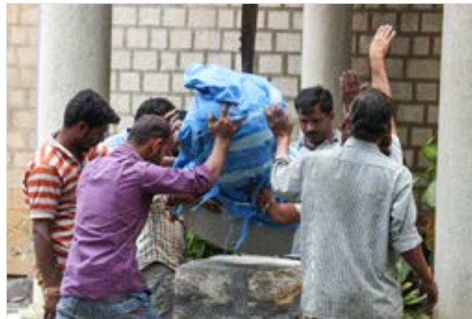
Installing the stone sculpture on the pedestal made up of stone and concrete.
