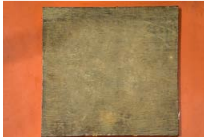
The required size of the MDF board is placed over the work area.
