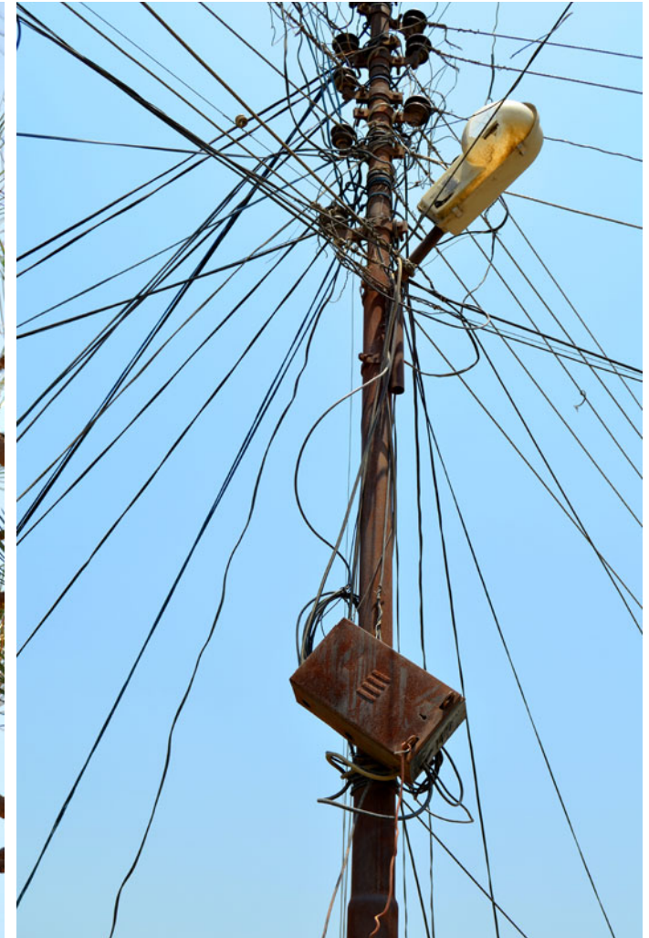
Wired chaos on an electric pole
