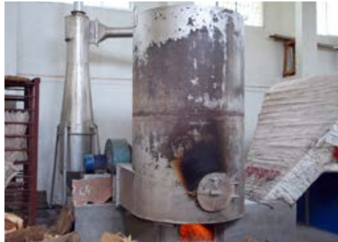
The furnace that is used to produce heat.
