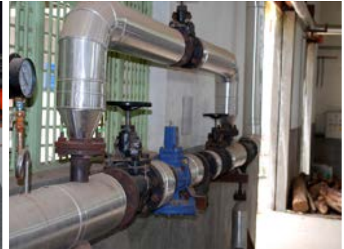
The pipe hose enables the transportation of heat for processing the cocoons.
