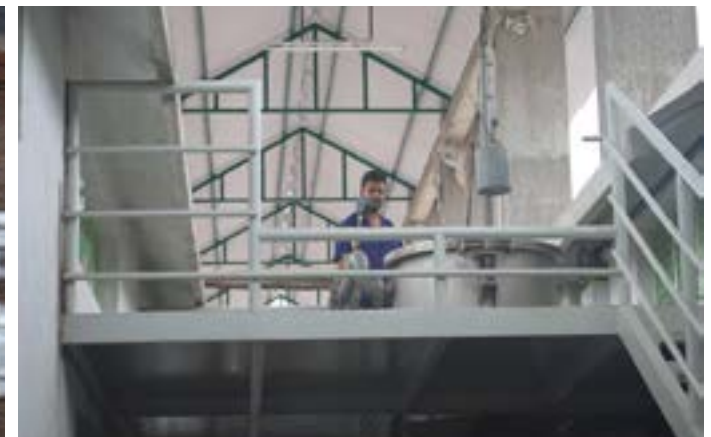
The boiler that enables the process of cocoon cooking.
