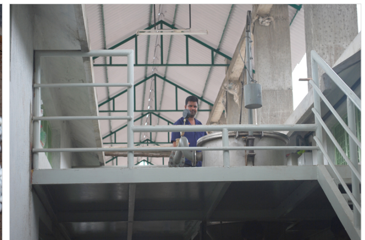
The boiler that enables the process of cocoon cooking.
